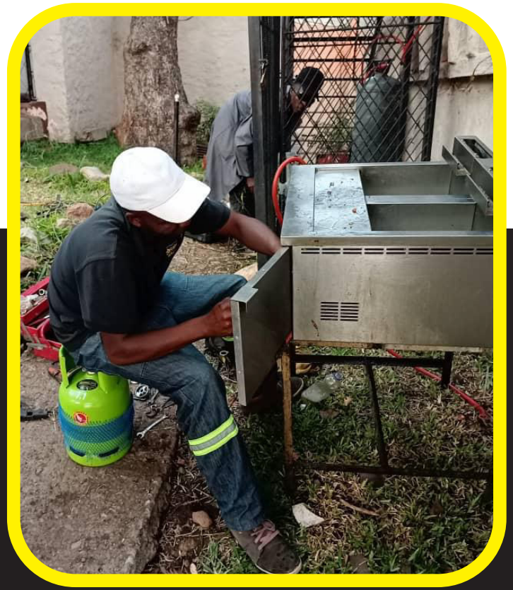
Carribea Bay Equipment Service
